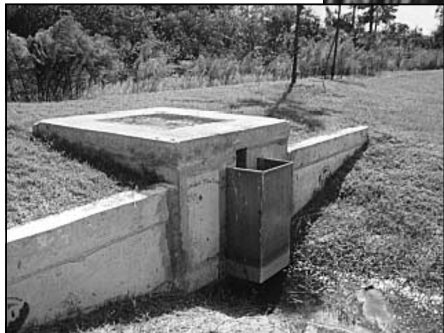
▲ Outflow Control Structure
