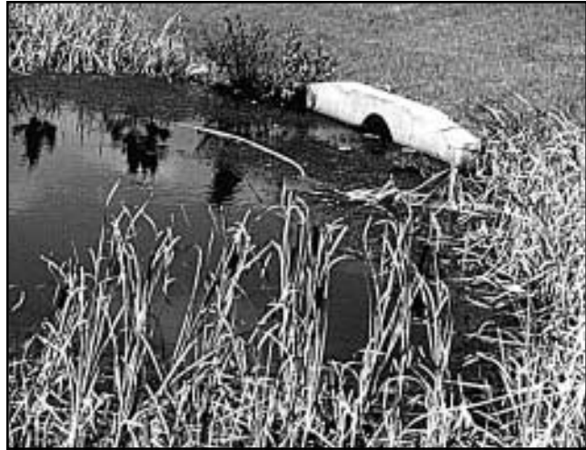
▲ Typical inflow pipe.
