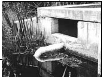
▲ Wet detention pond outfall structure.
